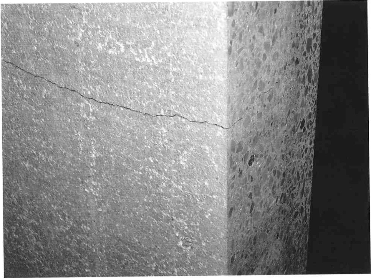
Horizontal Crack produced by DOE Pipe Missile
