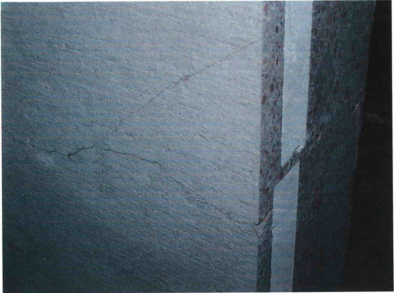
Cracking at right edge of panel backside
