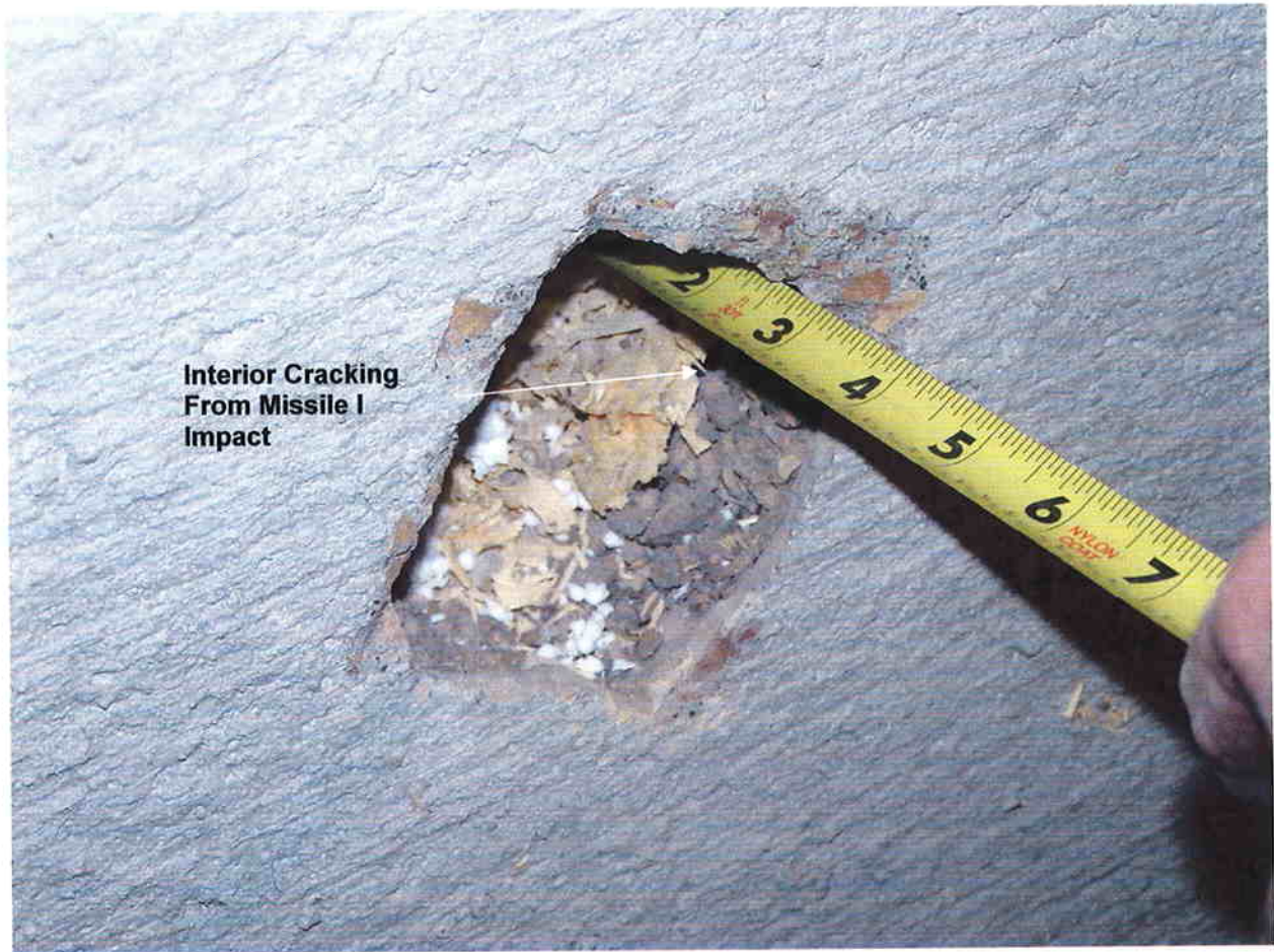
Panel penetration by Missile IV
